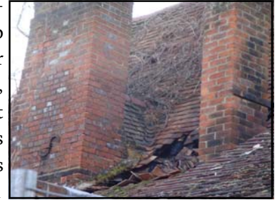
Fire damage to the Old Rectory's roof
